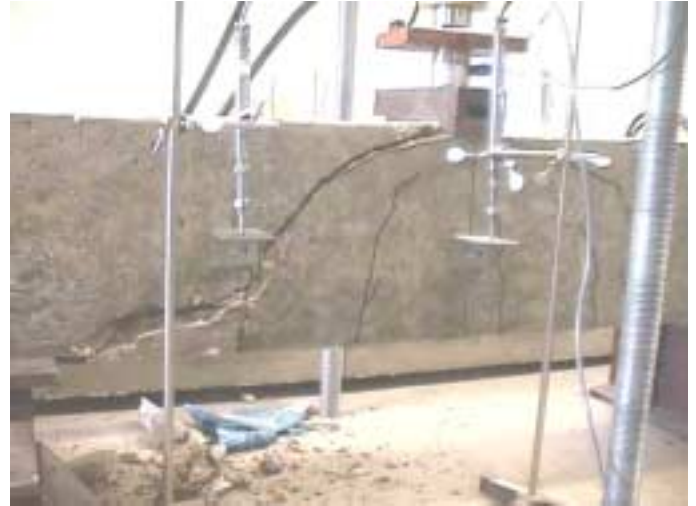
Figure 5: Shear failure (BM2).
