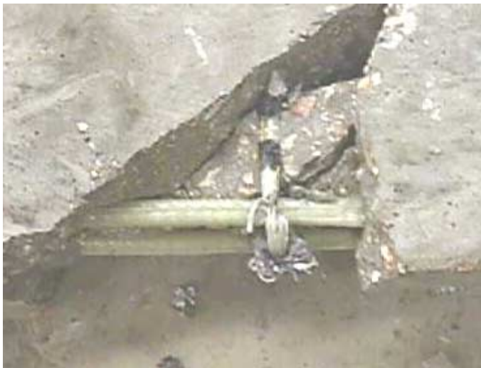
Figure 4: Rupture of GFRP stirrups
