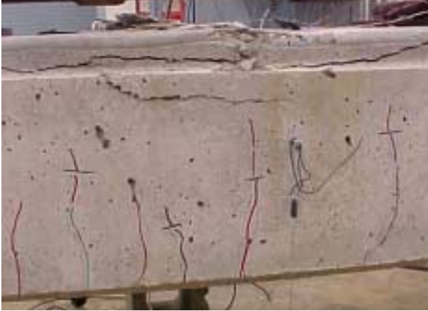
FIGURE 4 Failure of the steel-RC panel during the flexural testing.
