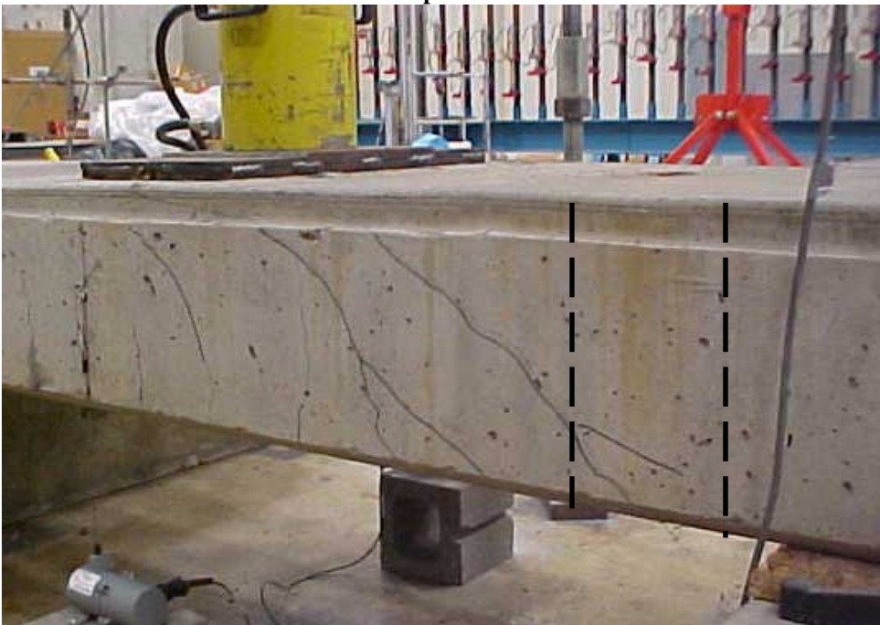
FIGURE 8 Shear failure of the FRP-RC panel.
