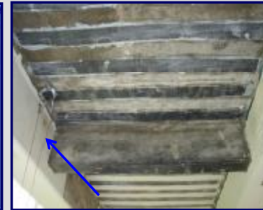
Damage Detection via Coaxial Crack Sensors
