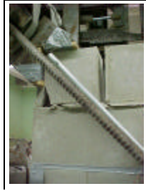
Figure 12. Splitting failure in wall WI 2
