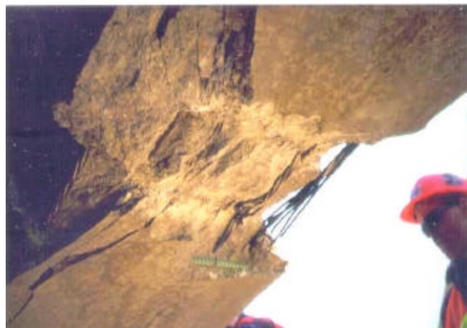
Figure 1. Fractured Tendons after the Removal of the Damaged Concrete
