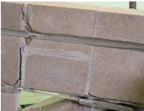
c) Splitting Cracks in the Embedding Material (CO2-GRE22)
