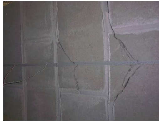
b) FRP Debonding: Formation of the 45° Cracks at the Head Joints (CO2-GRC31)
